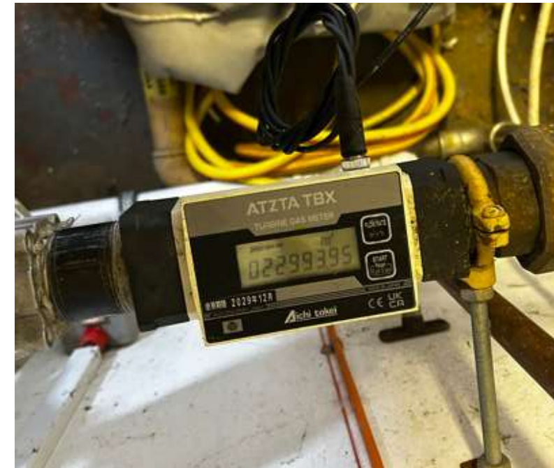
Existing Gas Submetering Trust HQ
