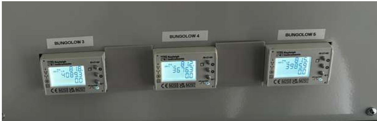
Existing Power Submetering at St Georges
